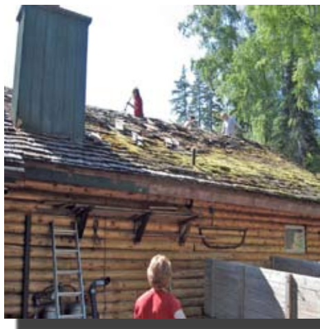
Volunteers from New Jersey and Colorado removing cedar shakes from a home on Big Lake.
